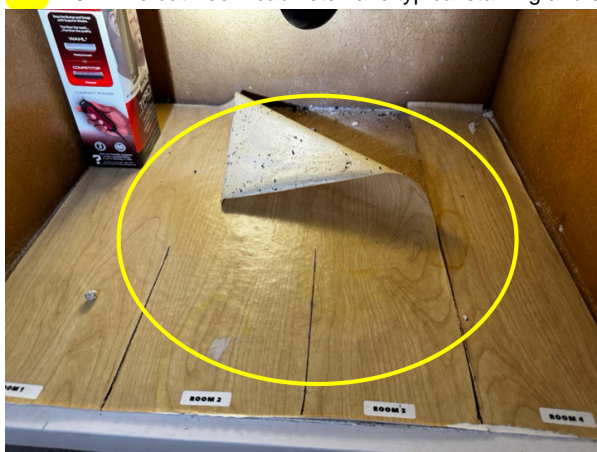
Example: staining/deterioration at north side hallway bathroom
