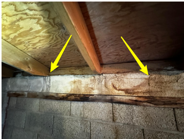
Example: moister staining
