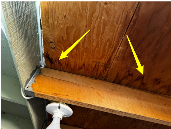
Example: moister staining
