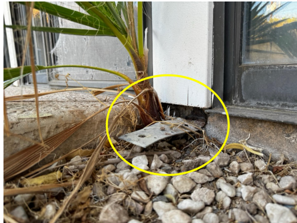
Example: unsecured wall anchor
