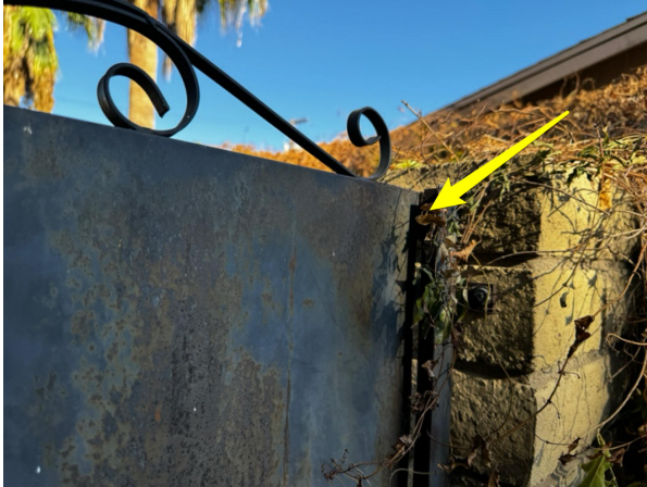
Example: gate does not close
