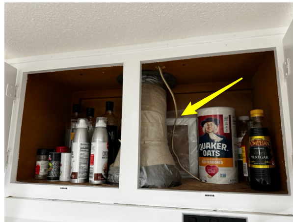
Example: exposed wiring
