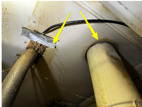
Example: moisture staining
