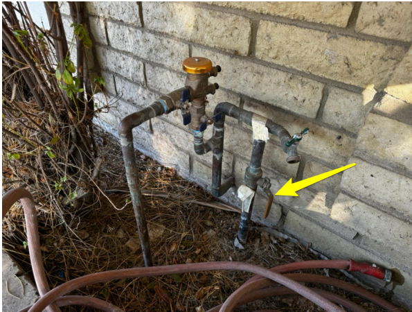
Main water shut off valve
