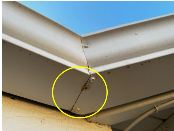
Example: evidence of leaking at seam
