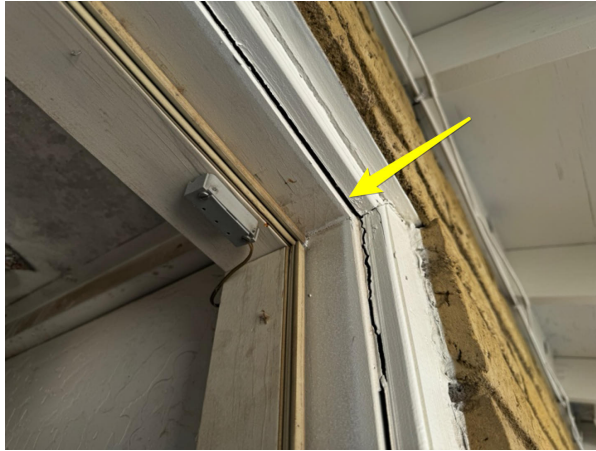
Example: various gaps/openings/separations
