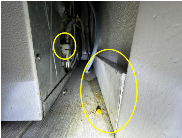
Leak & water damage
