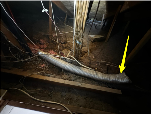
Example: incomplete installation
