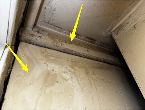
Example: moisture staining
