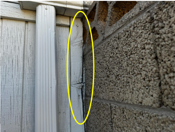
Example: rotted wood
