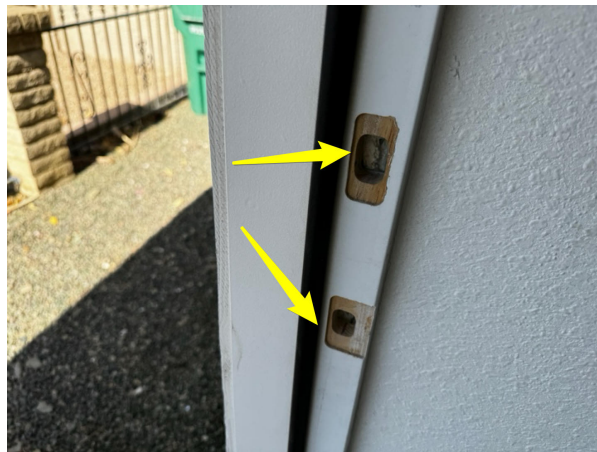
Example: missing strike plates at Room #9 door
