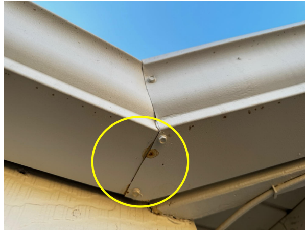
Example: evidence of leaking at seam
