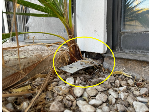
Example: unsecured wall anchor
