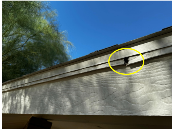
Example: damaged trim
