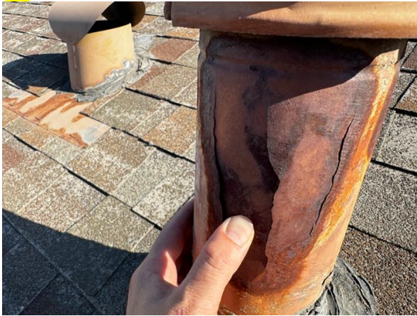
Example: rusted/damaged flue
