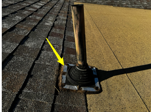
Example: plumbing vent roof jack improperly installed atop shingles
