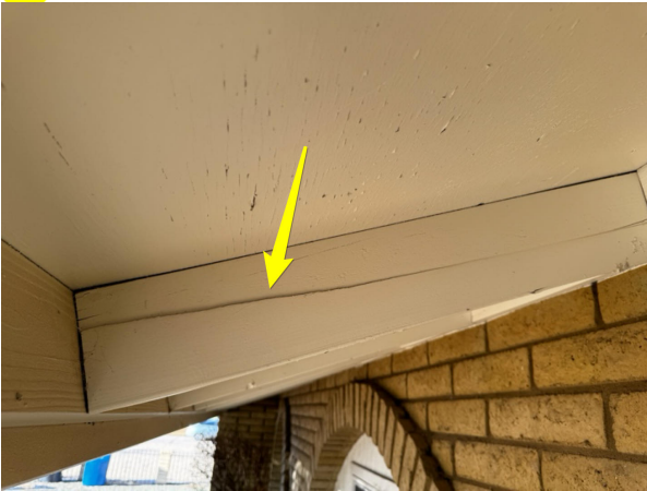
Example: cracked tail
