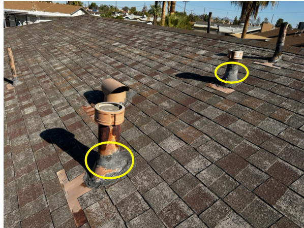
Example: storm collars not installed
