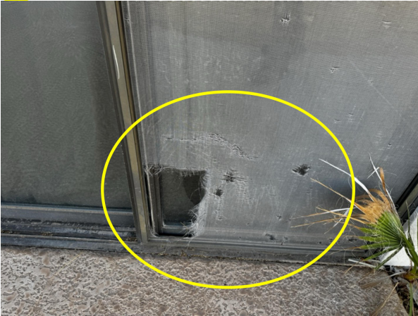
Example: damaged screen at rear patio door
