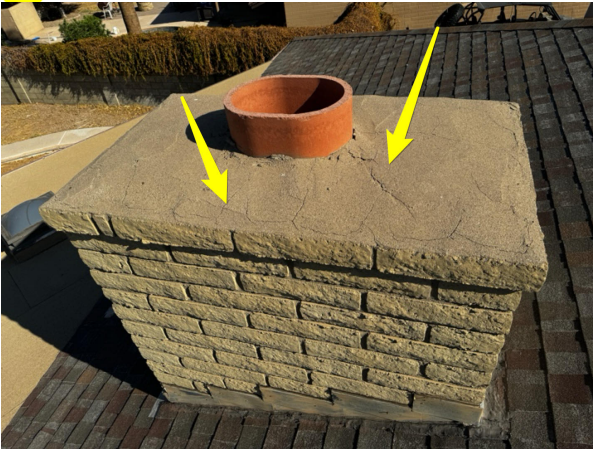
Example: cracks at crown
