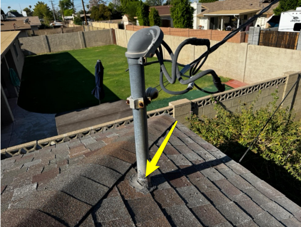
Example: no roof jack installed at electrical mast penetration
