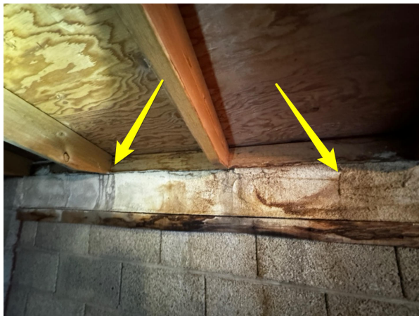
Example: moister staining
