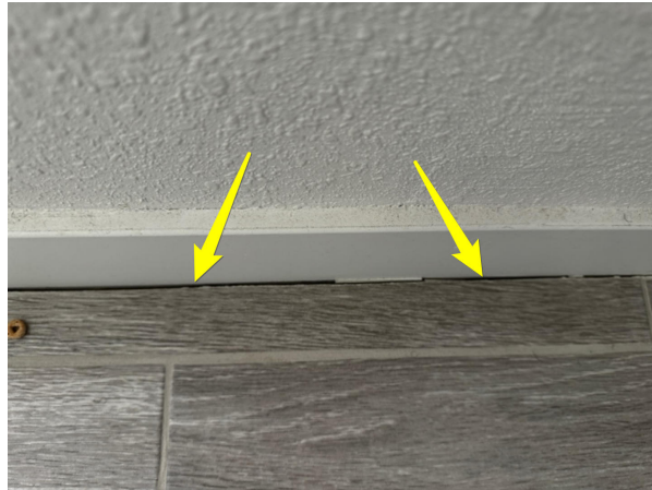
Example: damaged/incomplete grout
