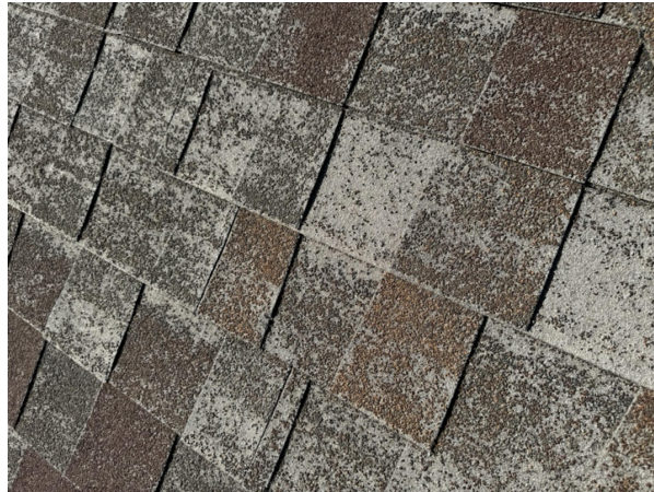
Example: significant granule loss
