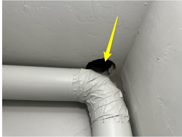
Example: hole in ceiling near dryer vent
