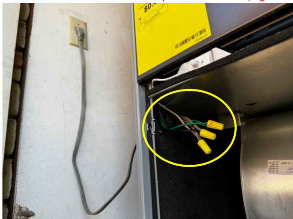
Exposed wiring connections
