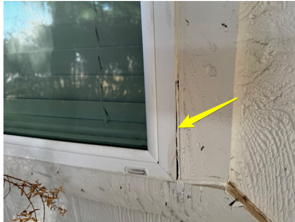
Example: various gaps/openings/separations
