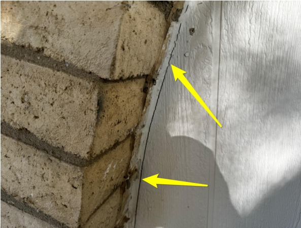
Example: various gaps/openings/separations
