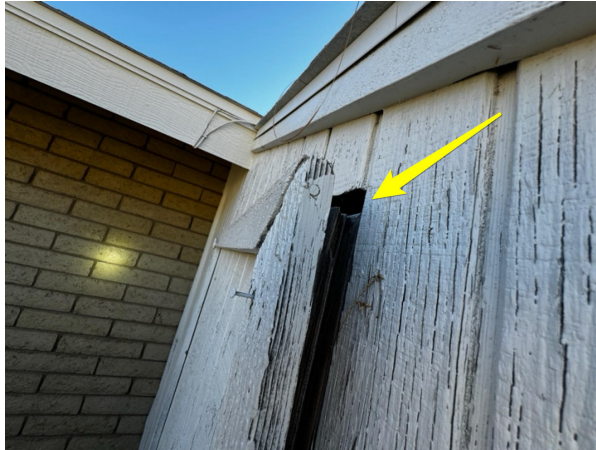
Example: door does not close/latch properly
