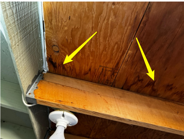
Example: moister staining
