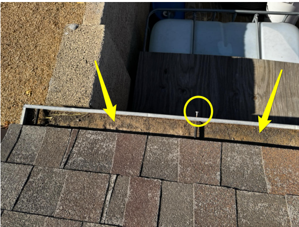
Example: gutter full of debris & loose anchor
