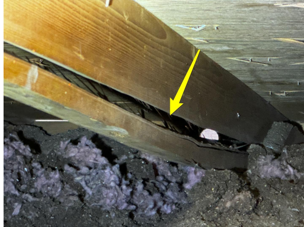
Example: cracked rafter
