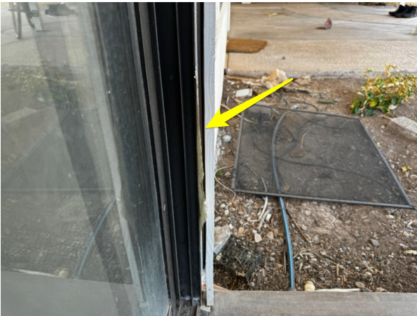
Example: various gaps/openings/separations
