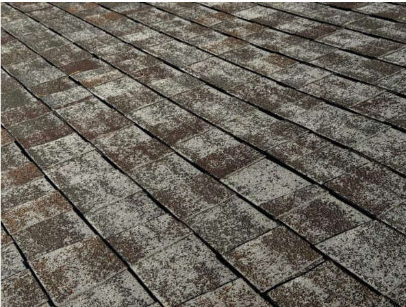
Example: significant granule loss
