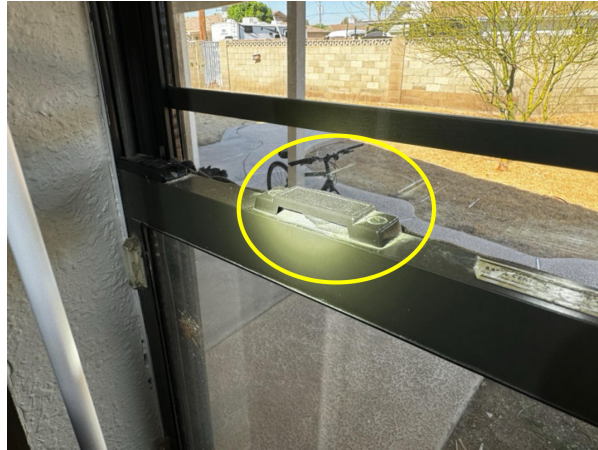
Example: damaged latch handle
