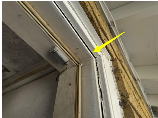
Example: various gaps/openings/separations
