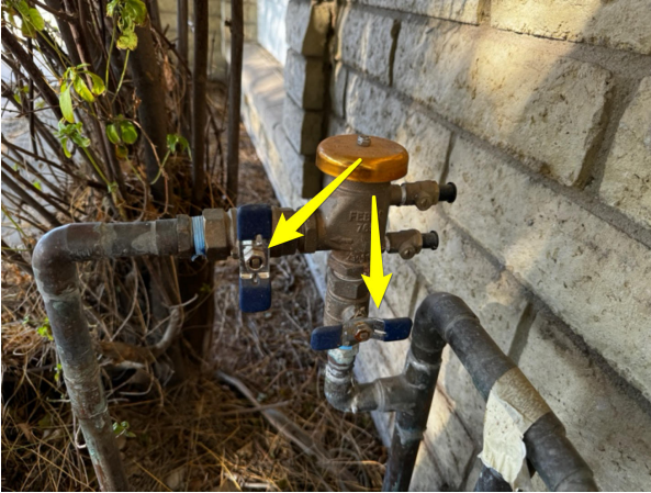
Water supply valves shut down
