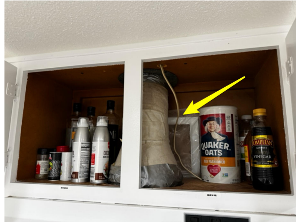
Example: exposed wiring
