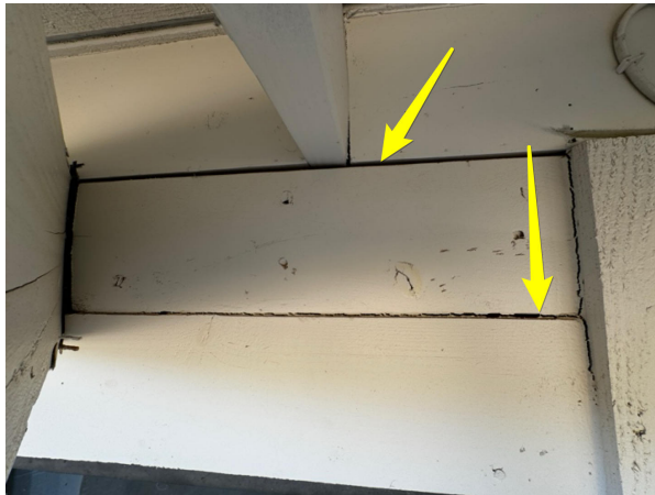
Example: various gaps/openings/separations
