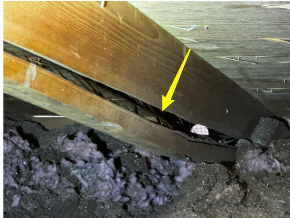
Example: cracked rafter
