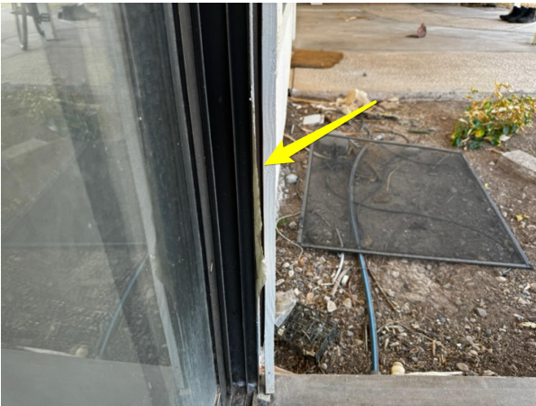
Example: various gaps/openings/separations
