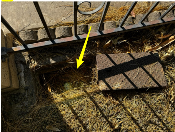
Debris in meter box
