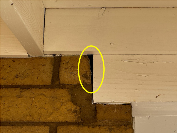
Example: various gaps/openings/separations
