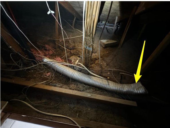
Example: incomplete installation
