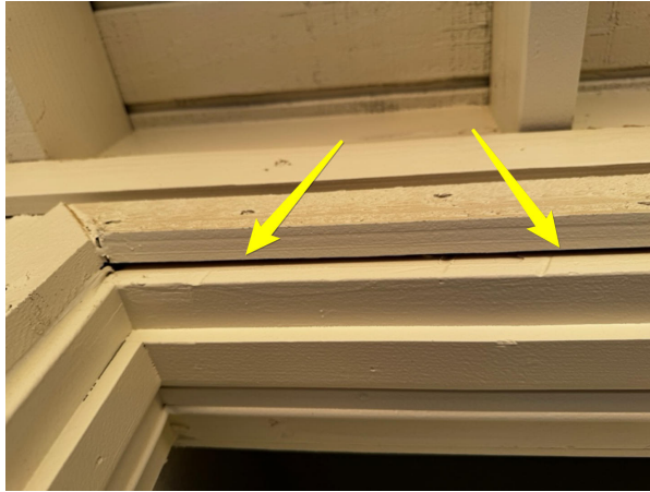
Example: various gaps/openings/separations
