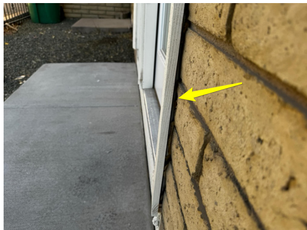
Example: various gaps/openings/separations
