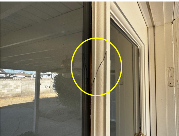
Example: damage at rear patio door trim
