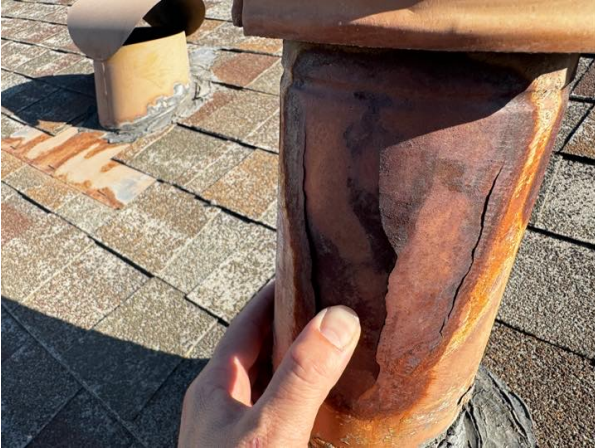
Example: rusted/damaged flue
