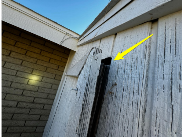
Example: door does not close/latch properly
