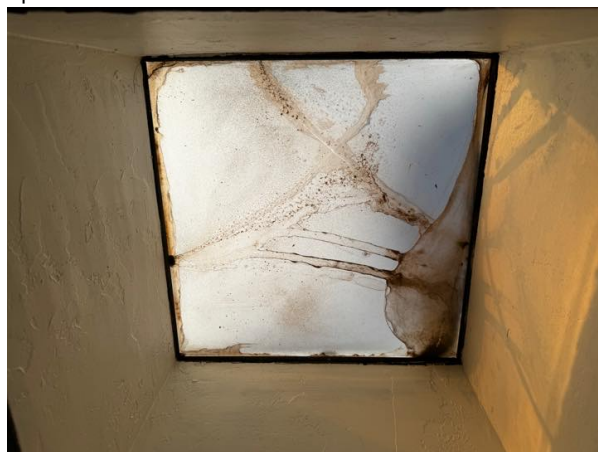
Evidence of past leaking
