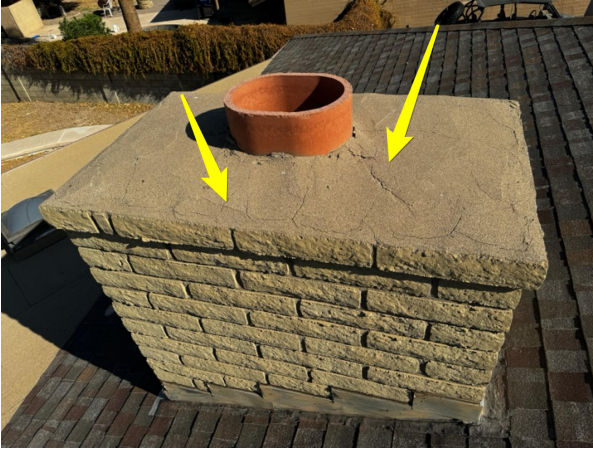
Example: cracks at crown
