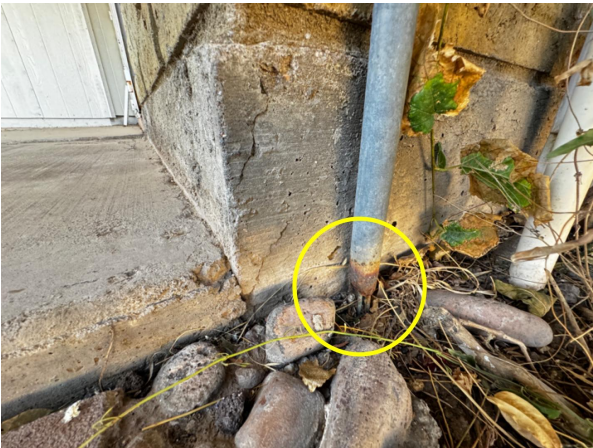
Damaged conduit & exposed wiring
