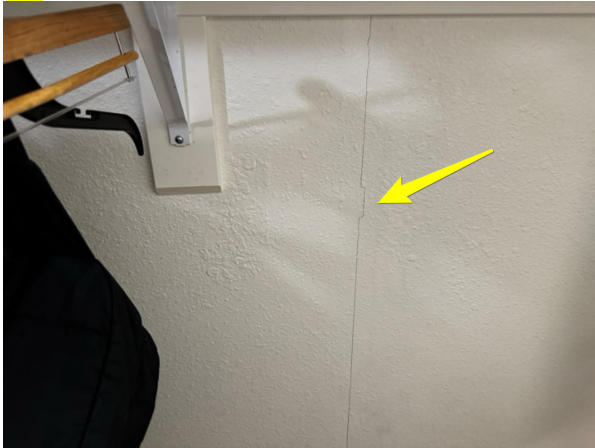
Example: crack in south bedroom closet
