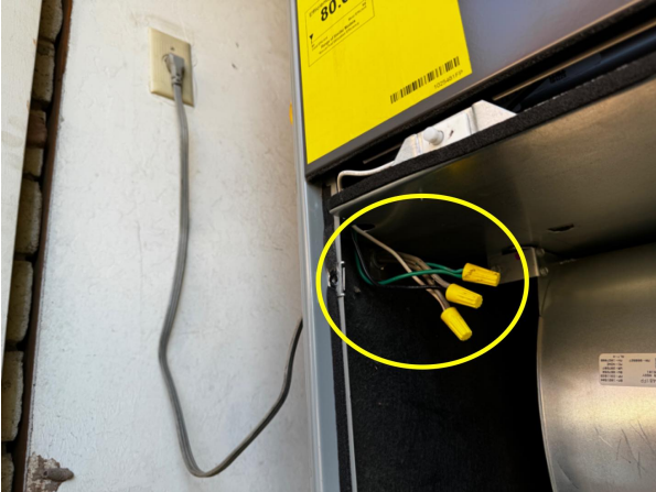
Exposed wiring connections
