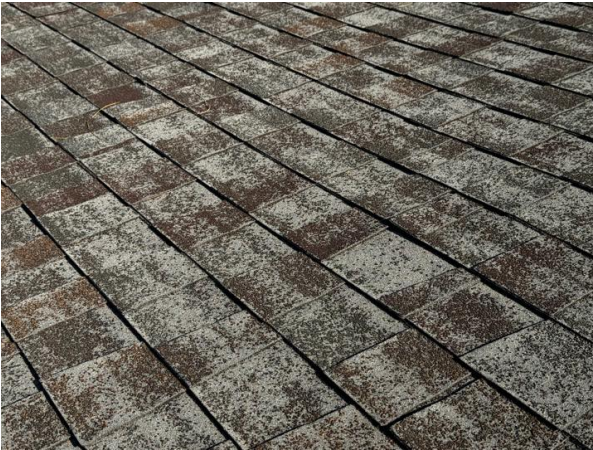
Example: significant granule loss
