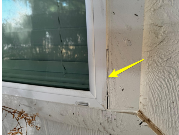
Example: various gaps/openings/separations
