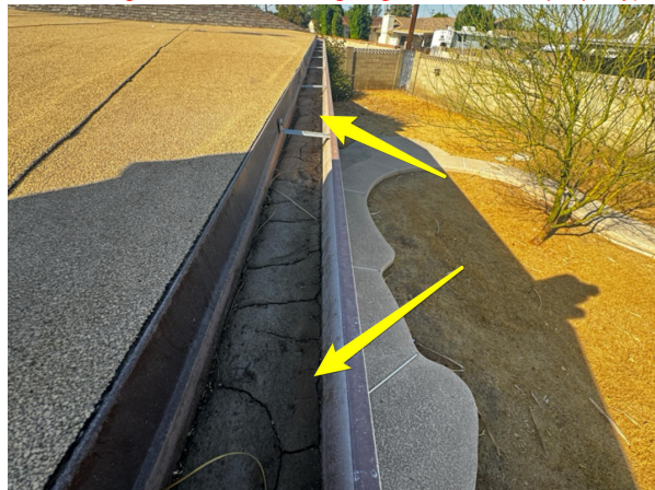
Example: gutter full of debris
