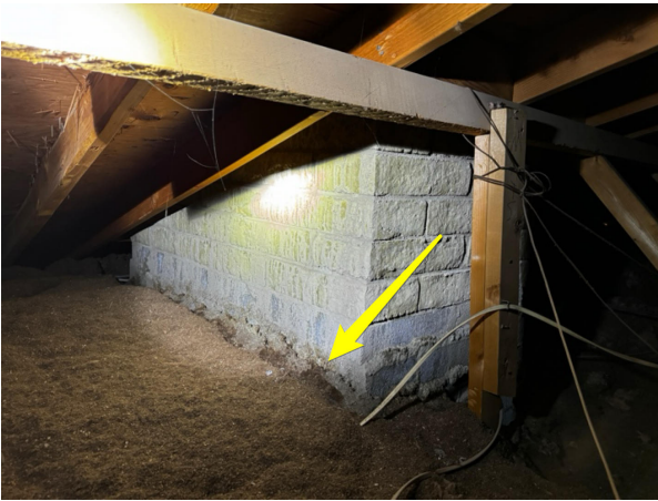
Example: moisture staining
