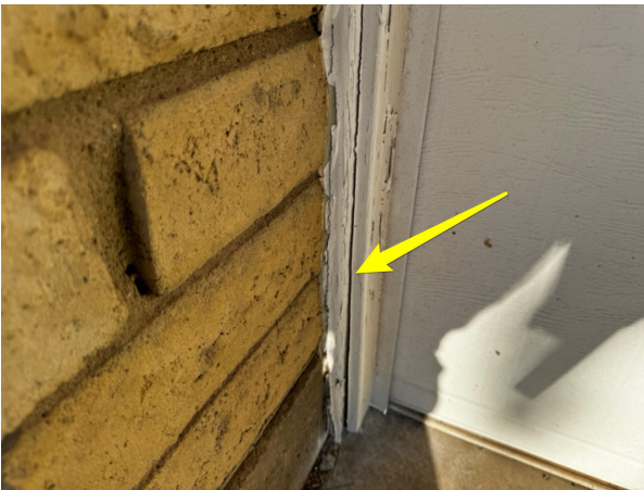
Example: various gaps/openings/separations
