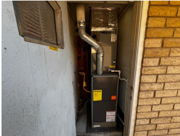
Furnace & air handler
