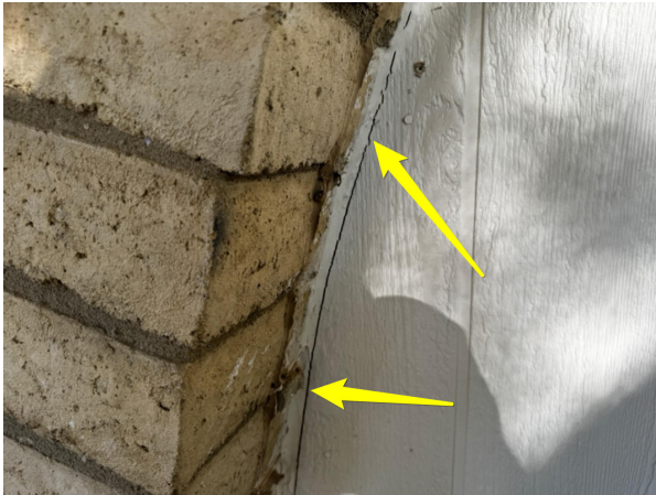
Example: various gaps/openings/separations
