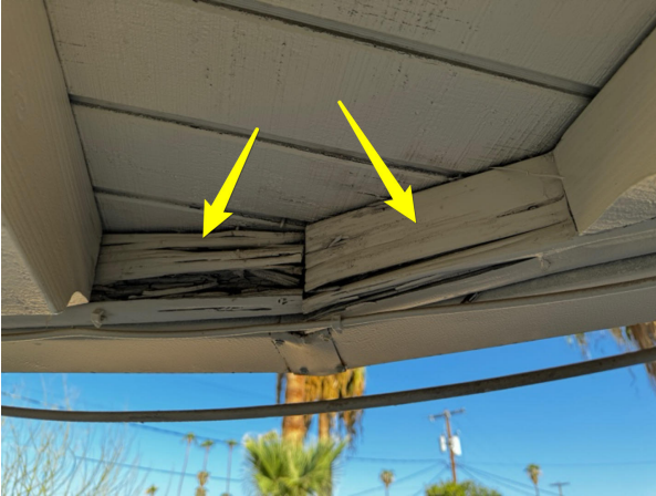
Example: rotted wood
