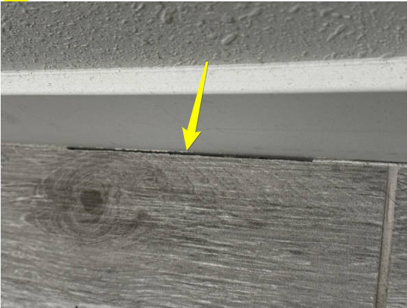
Example: damaged/incomplete grout
