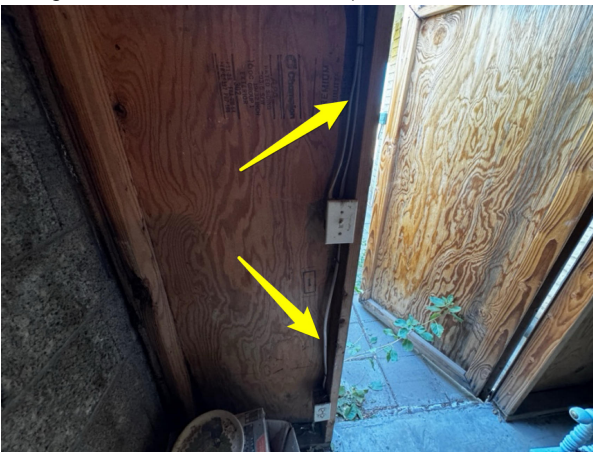
Example: exposed wiring
