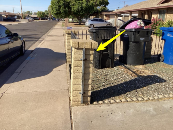
Example: loose/leaning column
