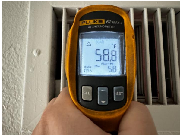
Supply temperature - South side system
