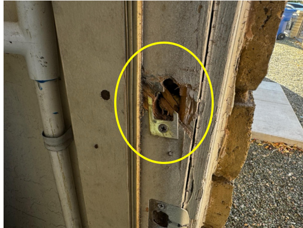
Example: damage at exterior closet door jamb
