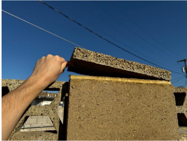
Example: loose column cap
