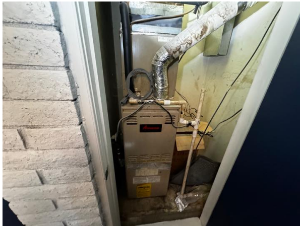
Furnace & air handler
