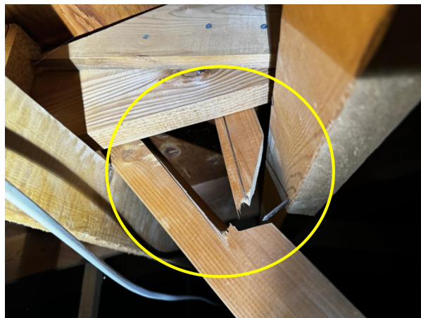
Example: loose framing
