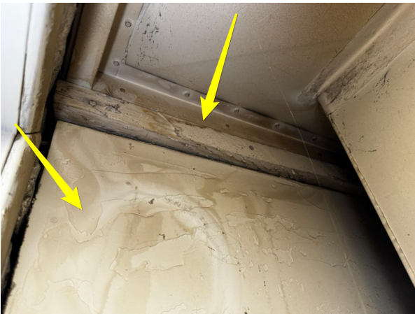
Example: moisture staining
