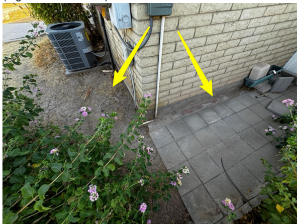
Example: evidence of water ponding
