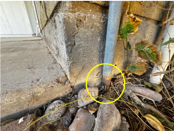
Damaged conduit & exposed wiring
