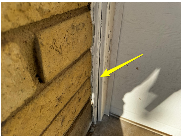
Example: various gaps/openings/separations
