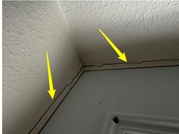
Example: separations at door & window perimeters
