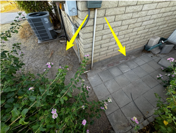
Example: evidence of water ponding
