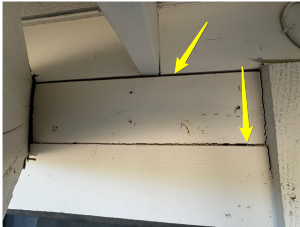
Example: various gaps/openings/separations
