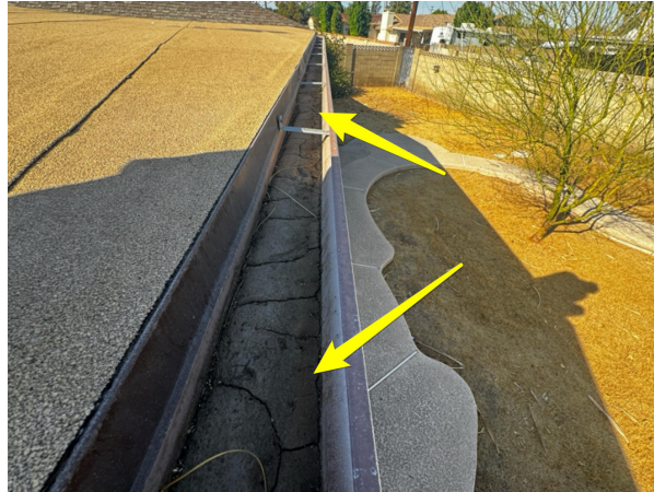
Example: gutter full of debris
