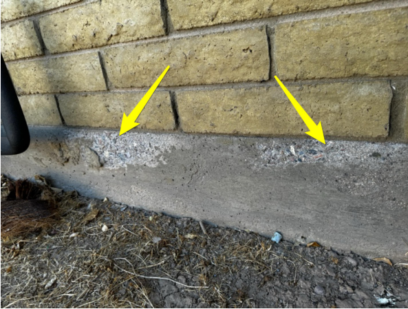
Example: surface deterioration
