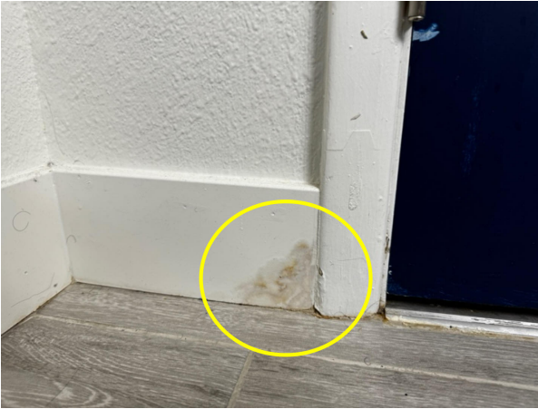
Example: staining at north hallway bathroom base trim
