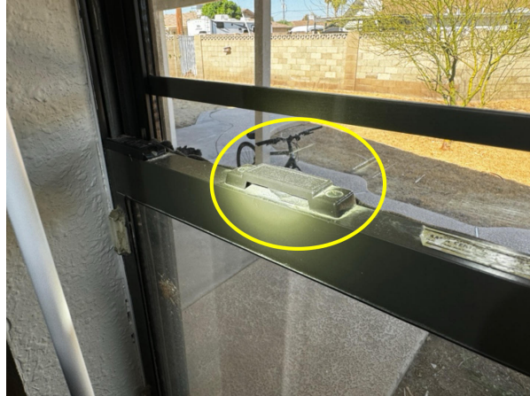
Example: damaged latch handle
