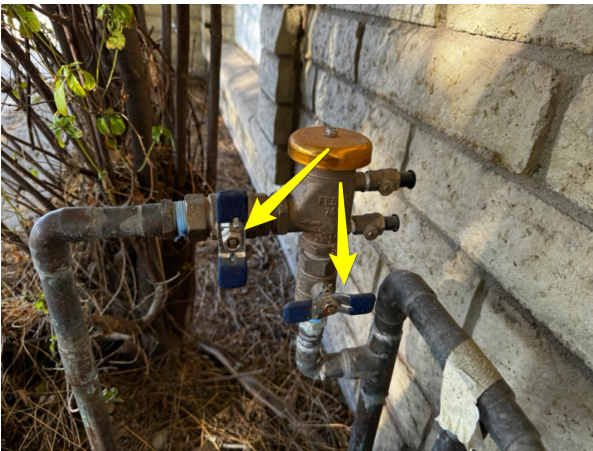
Water supply valves shut down
