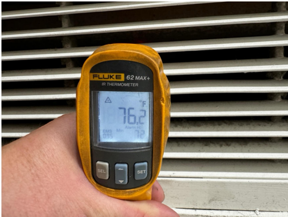
Return temperature - South side system
