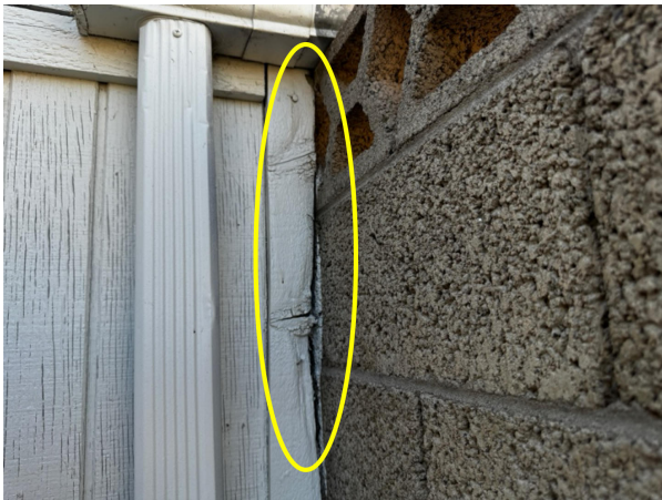
Example: rotted wood
