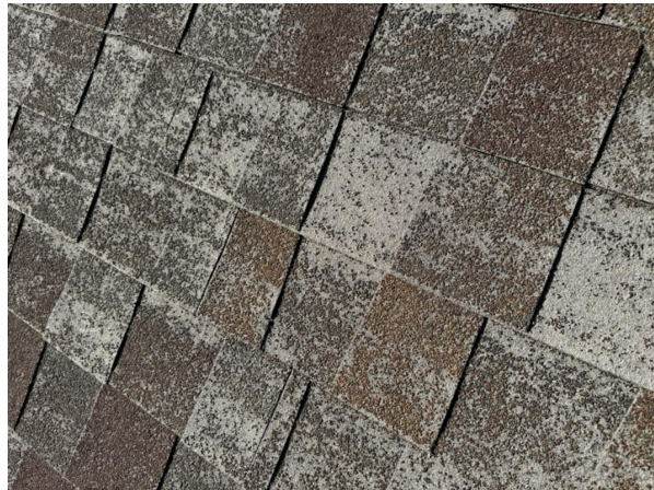
Example: significant granule loss
