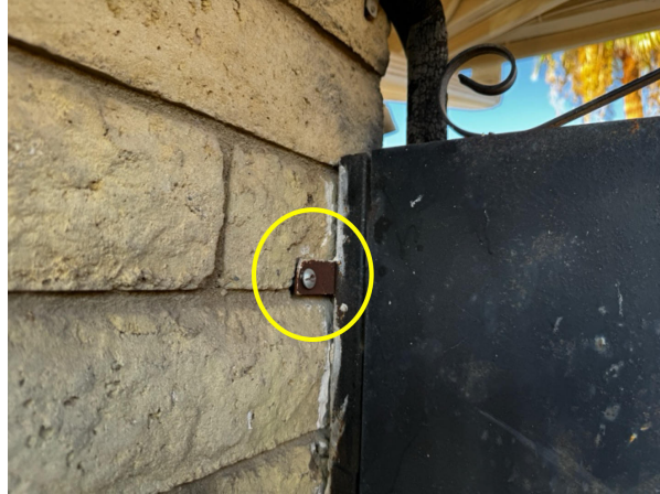
Example: loose anchor
