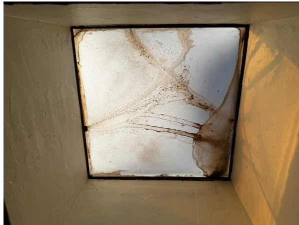
Evidence of past leaking
