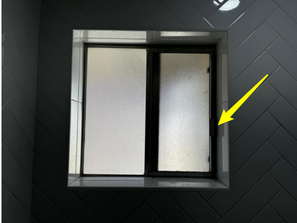
Example: window does not latch due to tile installation
