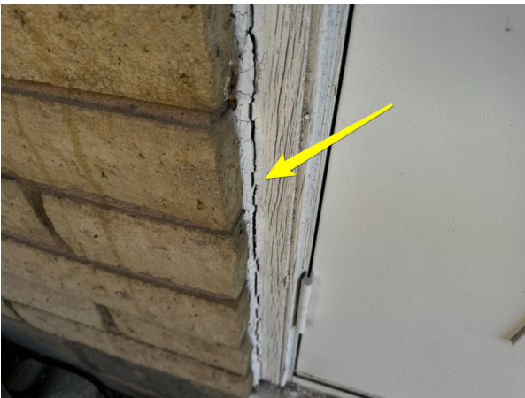
Example: various gaps/openings/separations
