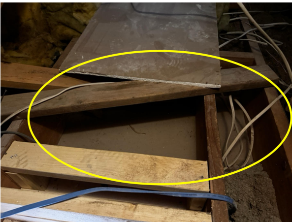
Example: missing insulation
