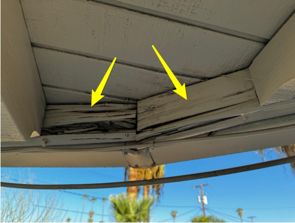
Example: rotted wood
