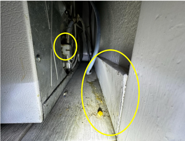
Leak & water damage
