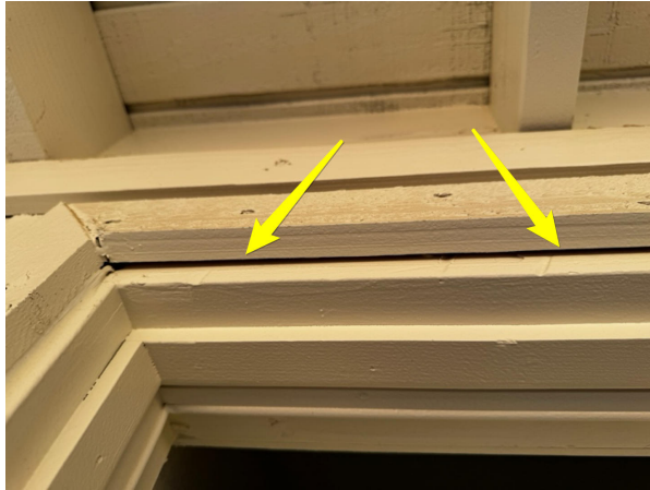
Example: various gaps/openings/separations
