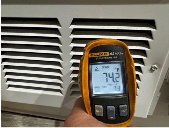
Return temperature - North side system
