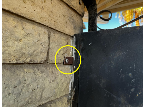
Example: loose anchor
