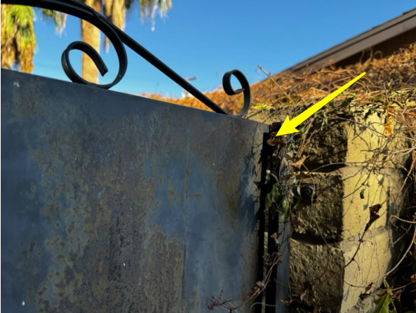
Example: gate does not close
