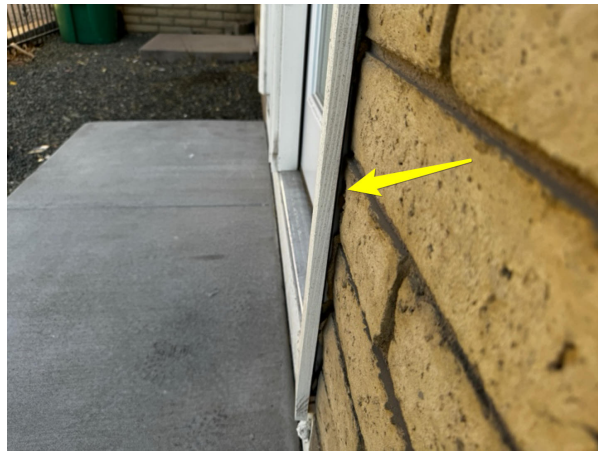
Example: various gaps/openings/separations
