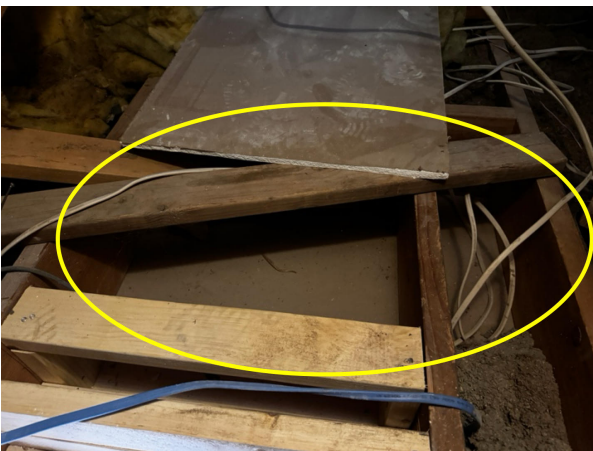
Example: missing insulation
