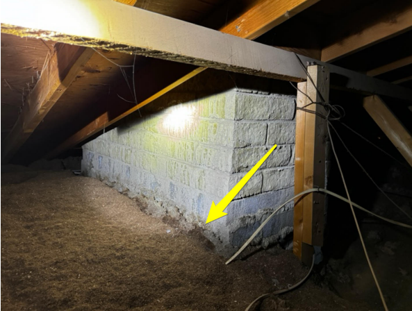
Example: moisture staining
