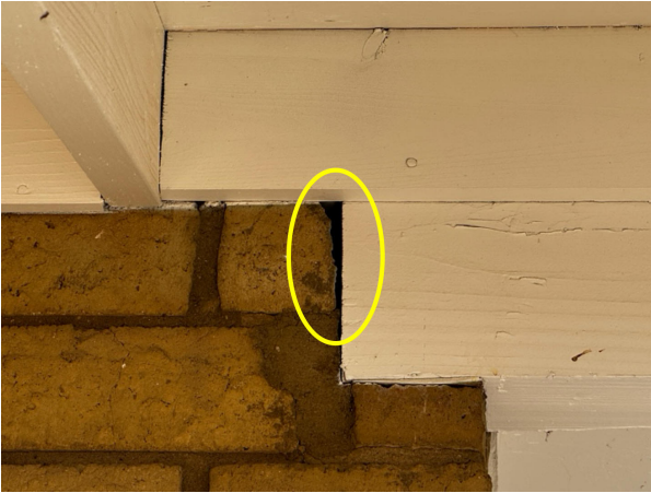
Example: various gaps/openings/separations
