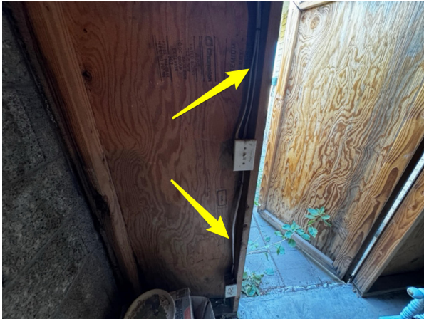
Example: exposed wiring
